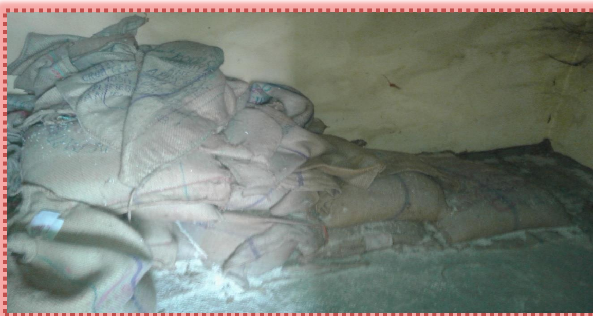
MDM : Storage food grains in additional classroom , not in proper way
